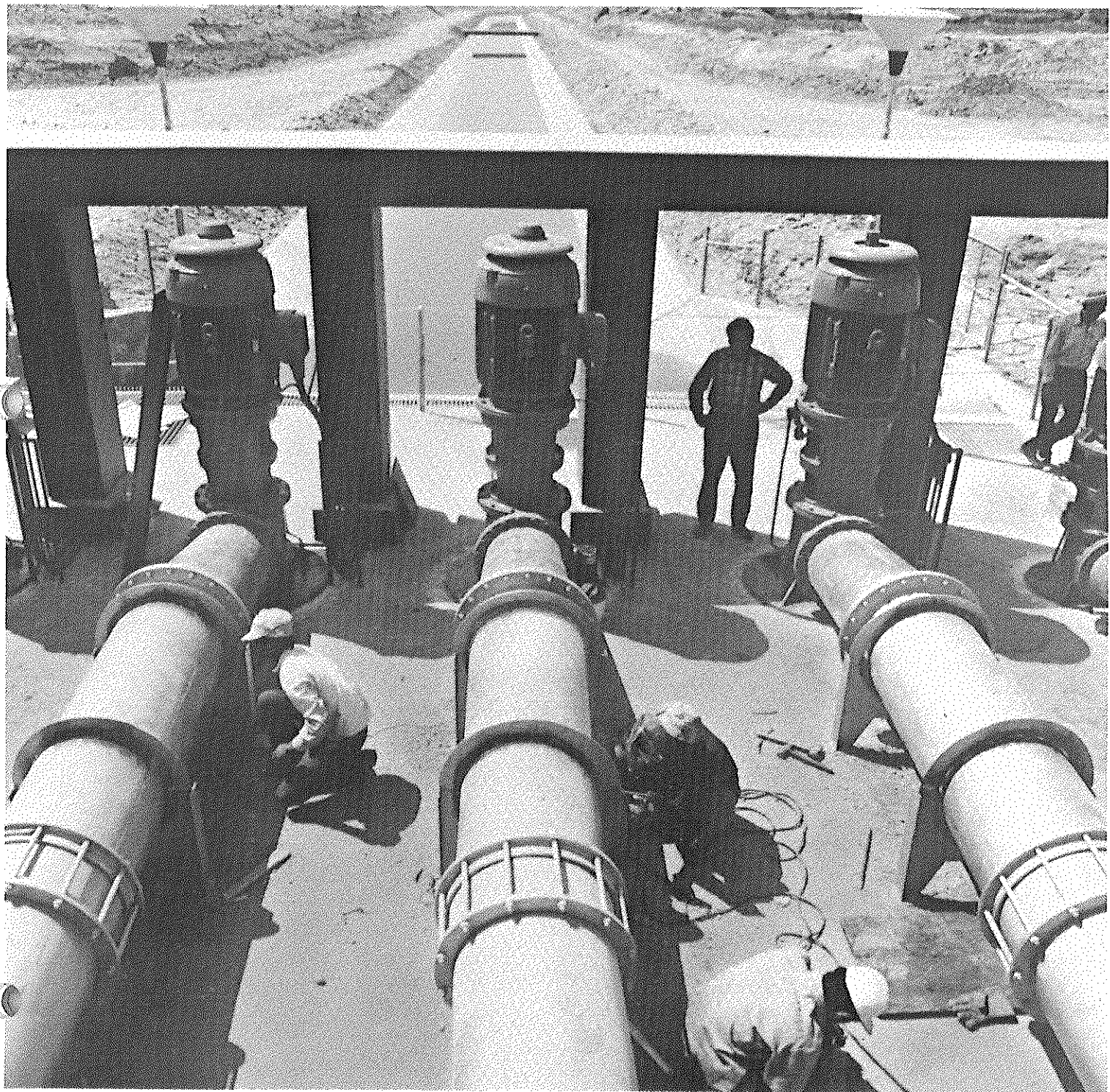
A modern pumping station in Iran, part of a multi-purpose development project designed to bring water, electric power and flood control to a populated river basin area.
